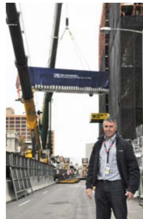
Professor David Smart on site during construction of the new diving and hyperbaric medicine facility in Hobart.
