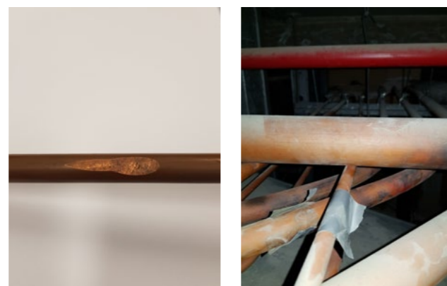
Figure 2 and 3: Vibrating waste pipe rubbing against N 2 O pipe (arrow) causing second large leak.
